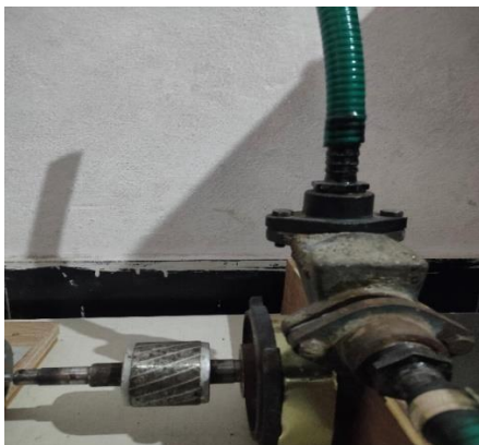
Fig-9: Motor and pump setup
